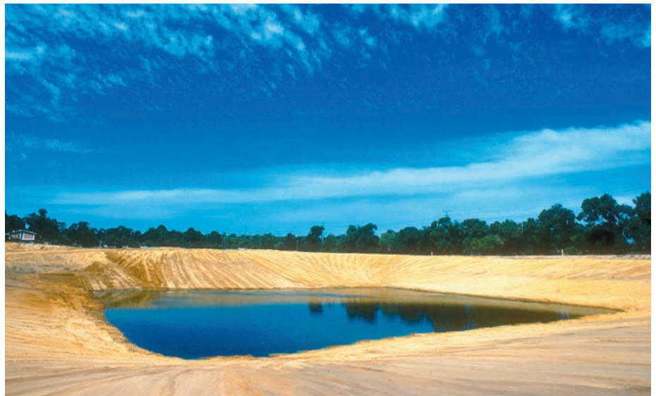
A newly excavated sewage treatment dam near Perth. Most endocrine disrupting chemicals in Australia's environment come from domestic sources and are not fully removed by the sewage treatment process. Willem van Aken
