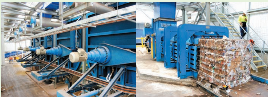
Left: German made ISKA® Percolation machines clean and deodorise the organic garbage components generating renewable energy and quality compost. Right: Valuable quantities of retrieved, recyclable paper and cardboard product get sold on from the UR-3R facility. Global Renewables
