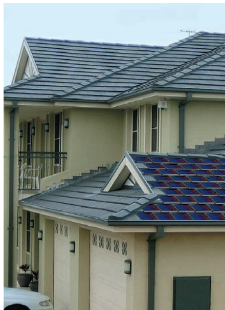
KISSTiles in place on the northern roof of a suburban home. Courtesy of Australian Design Awards
