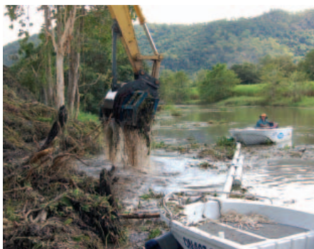
The excavator claws weeds from the water with the help of two small boats. Vern Veitch
