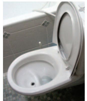
A trial of urine-separation toilets is currently underway in Queensland.
