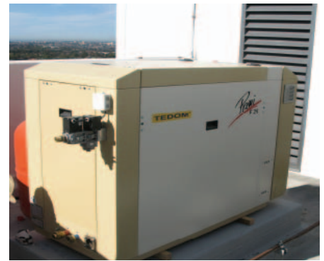
This 'cogen' gas generator, installed on an apartment tower in NSW, produces both electricity to serve some of the building's common areas and also approximately 50 kW of heat for domestic hot water. Conventional power stations, remote from the city, waste much of their heat. Kinesis Pty Ltd.
