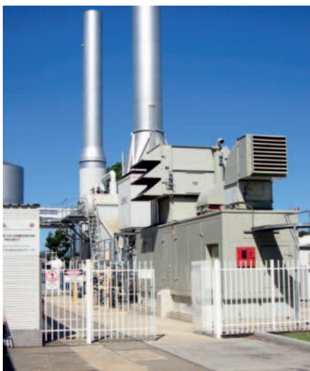
Coopers Brewery's on-site electricity cogeneration plant has saved 15 000 tonnes in annual greenhouse emissions. Coopers Brewery Ltd.
