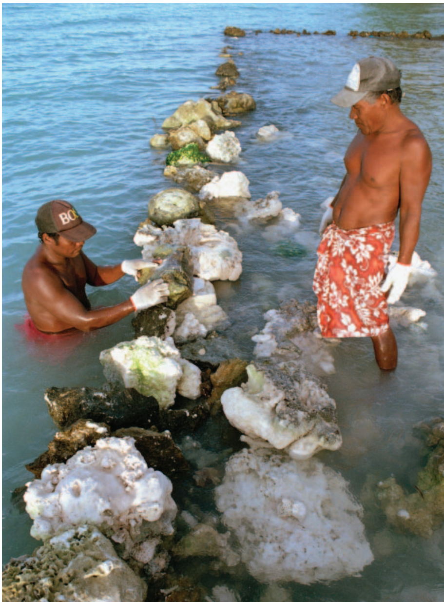
Kiribati men use coral blocks to build a retaining wall near their homes at the water's edge on Tarawa atoll, Kiribati. Such barriers could be contributing to shoreline erosion, rather than preventing it. J. Carlin/Panos
