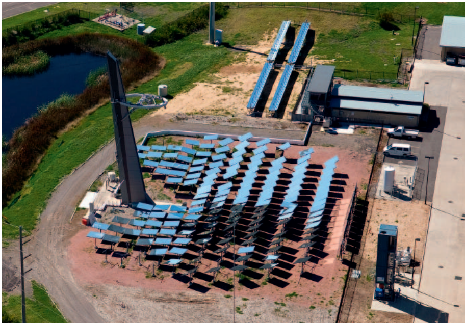
The National Solar Energy Centre, at CSIRO's facility in Newcastle, hosts a solar array tower and linear trough solar array. Nick Pittas, CSIRO
