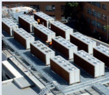
The main Royal Women's Hospital building in Melbourne is now cooled by 3C units. Muller Industries Australia
