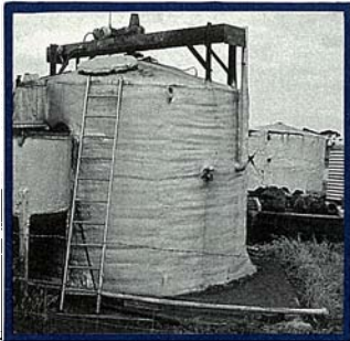
The pilot digester.
