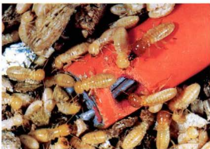
The soft insulating sheath of this cable has succumbed to giant termite ( Mastotermes darwiniensis ) soldiers and workers.
