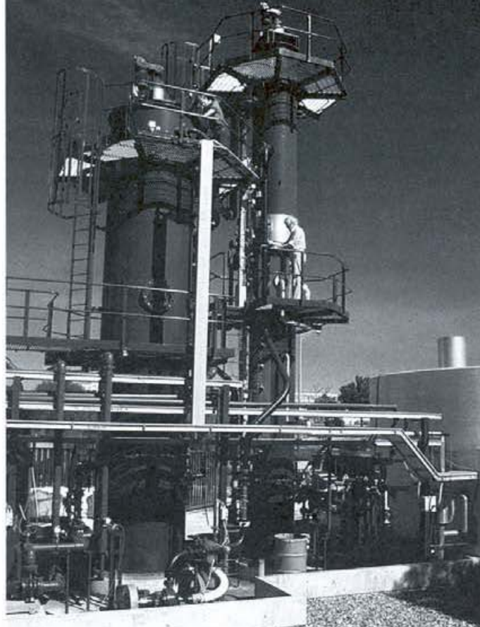
The continuous Sirotherm desalination plant at Leederville, W.A. Its twin columns (adsorber on the left, hot regenerator on the right) can treat 1 ML a day.
