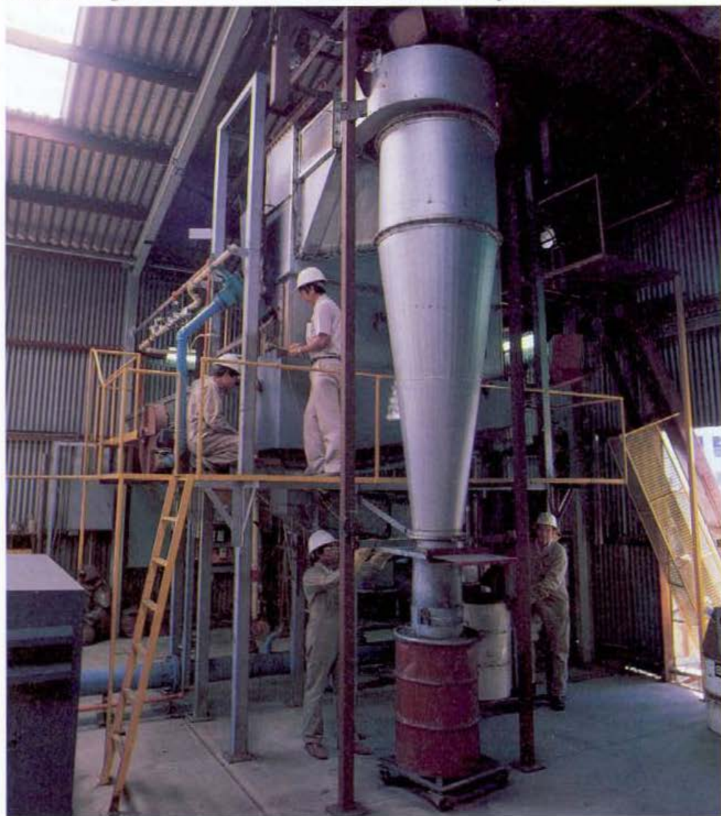
Below: Making charcoal in the Division's fluidised-bed combustion plant.
